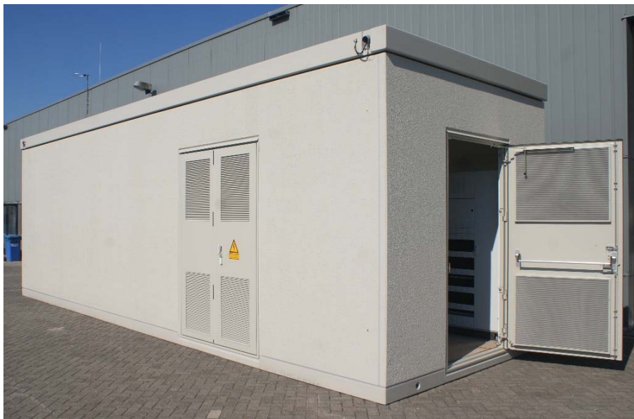
Figure 4: 1 MW DC distribution station
