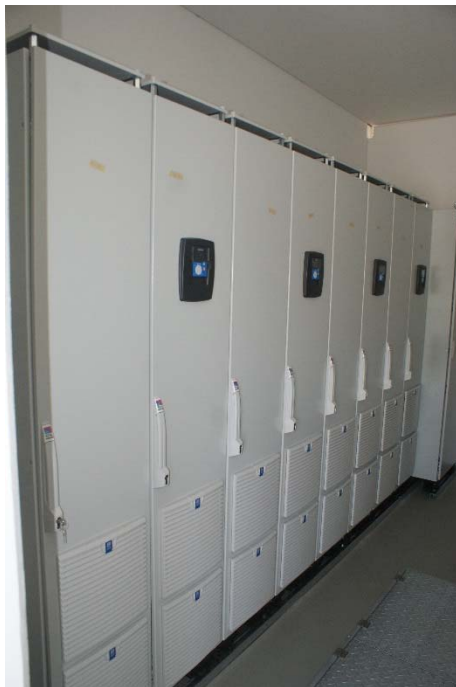
Figure 13: AFE converter panel
